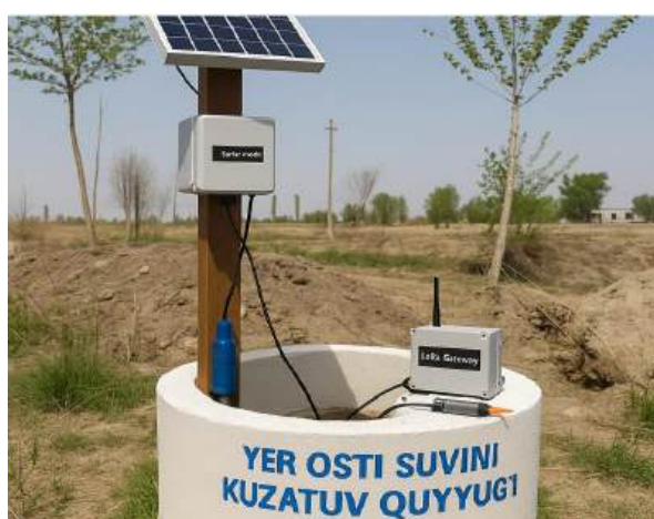
Figure 3. General view and placement of the device installed in the field
